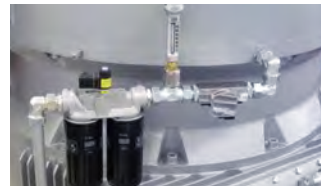
Oil filter with flow meter
