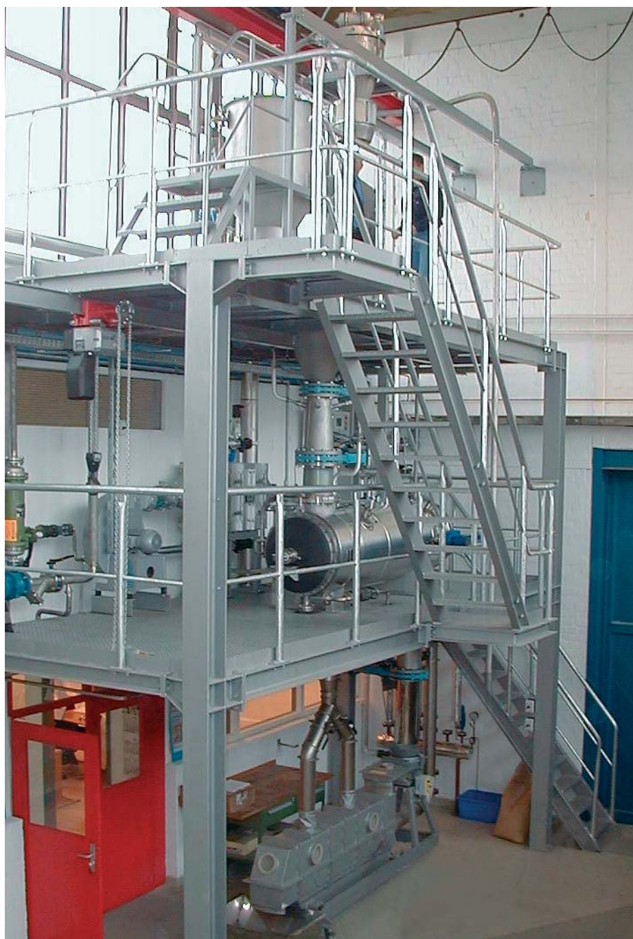
Hydrothermal cooking plant in the KAHL pilot plant at Reinbek
